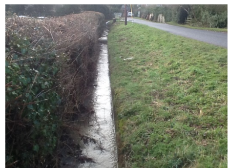
Narrow ditch at the northern end of Friday Street. The main route for all the run off from the village and all of the farmland upstream
